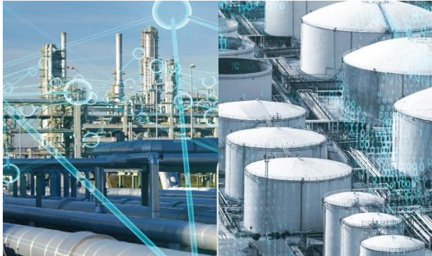
Onshore piping on plants & terminals
